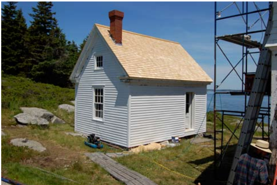
The School House with a new roof. It will house course instructors.
